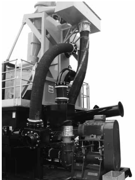
Rubber lined sealed slurry transfer pipes complete with heavy duty clamps
